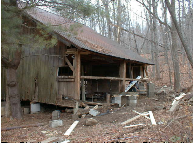
The building that housed the White Pine Healing Arts clinic and institute was a broken down barn
